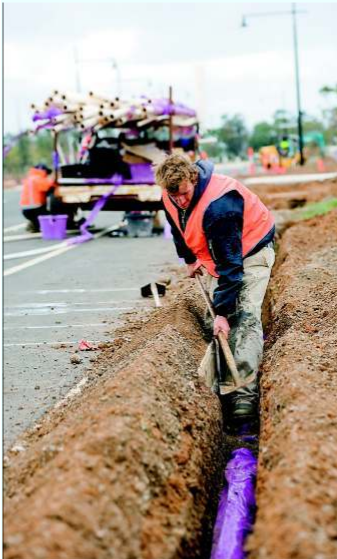
Laying it down: workers install purple piping to denote recycled water at the Eynesbury Township development.
